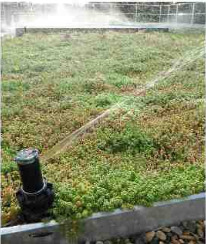
Spray irrigation on a green roof (Source: VEgetal i.D., 2019)
