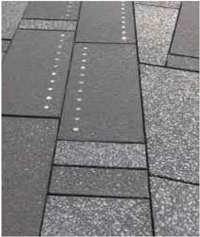
Natural stone paving
