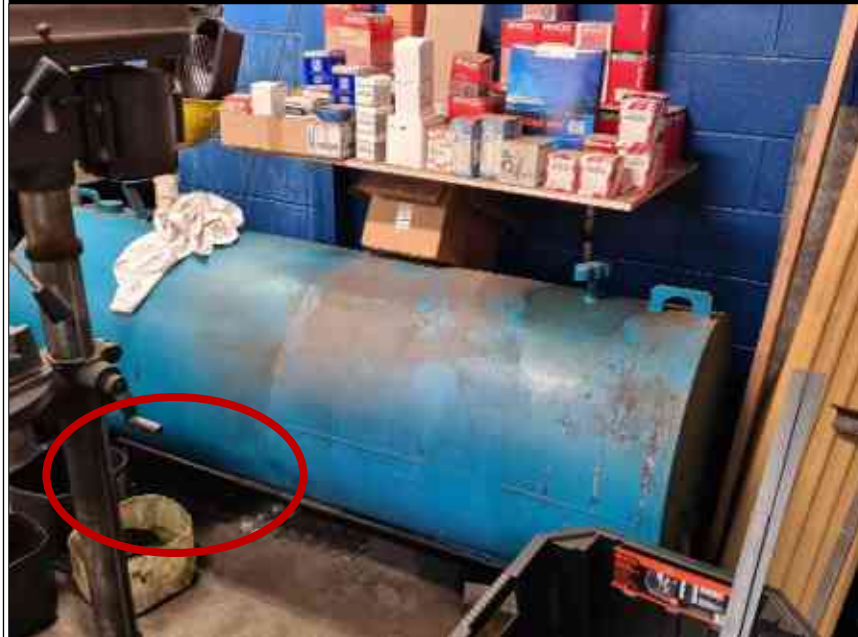
PHOTOGRAPH 4: AST WITH STAINING
