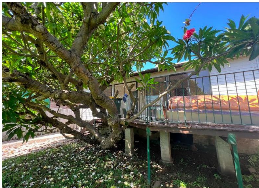
Figure 25 – Rear deck to be replaced, tree to be removed, view looking southeast (Source: 3+1 Heritage, 2023)
