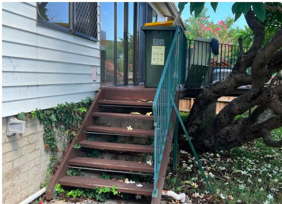
Figure 24 – Timber deck to be replaced, tree to be removed, view looking south (Source: 3+1 Heritage, 2023)
