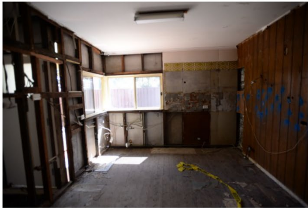
Image A10 View looking south at the dilapidated kitchen. The condition of the house is as the owners recently purchased it. The illegal work was done by the previous owners.
