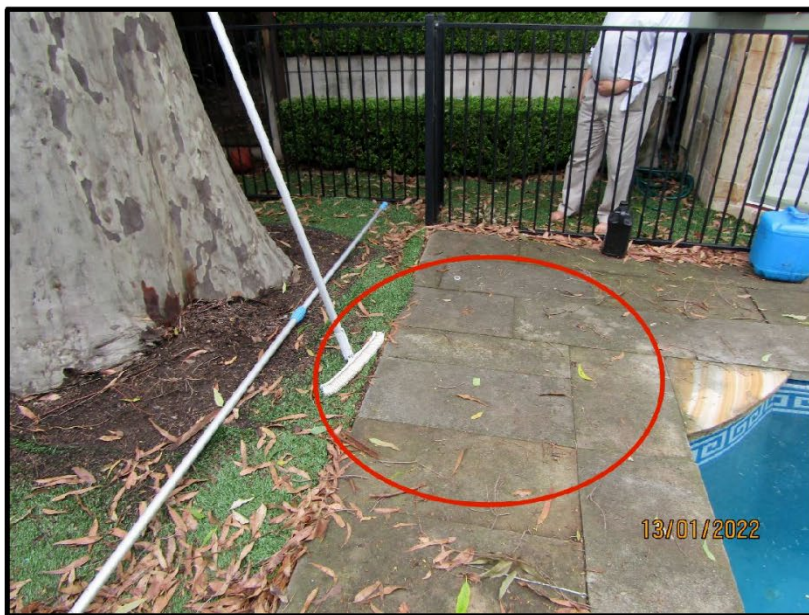
Figure 9: Spotted Gum's structural roots lifting the flag stones around the swimming pool edge
