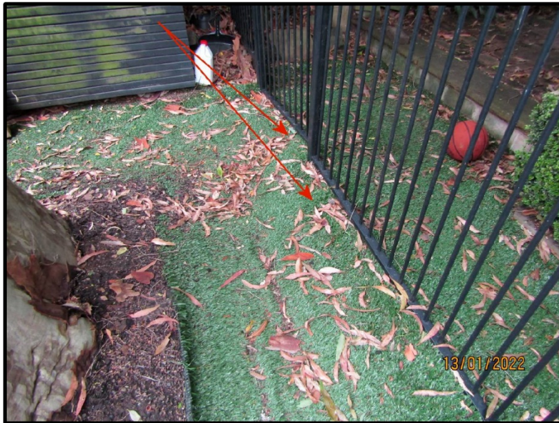
Figure 10: Showing the Spotted Gum's structural roots starting to lift the pool safety fence and interfering with the operation of the gate.
