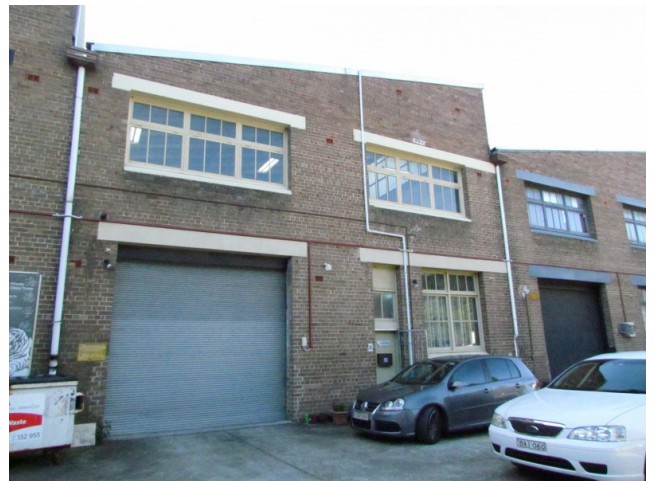
West façade of typical saw tooth roof factory bay remains relatively intact.
