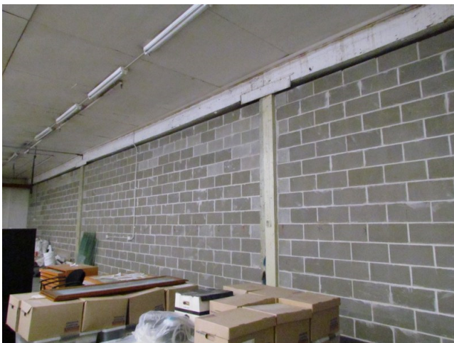
Lower level unit, with original timber supporting posts & beams incorporated into the later block dividing walls
