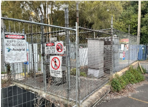
View of electricity substation Looking Southwest Inspected 15.06.2022
