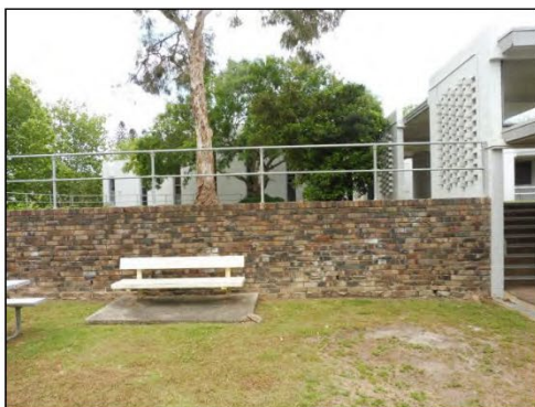
Figure 3.25 The proposed new ramp will require a small modification to the existing brick retaining wall (top of wall mid right). B105 is partially visible beyond.
