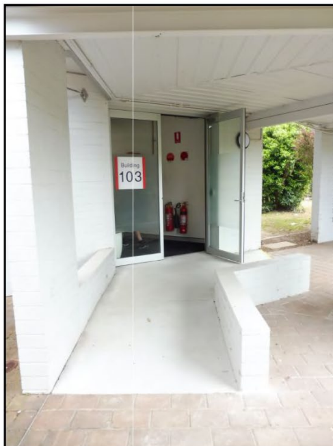
Figure 3.19 An existing access ramp and dwarf wall added to an entry of B103.
