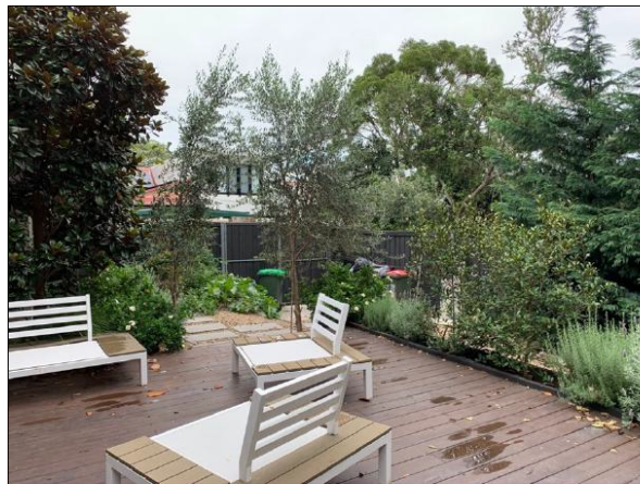
Figure 10: Timber deck on the western side of the building, looking towards the south western corner where it is proposed to construct the garage.
