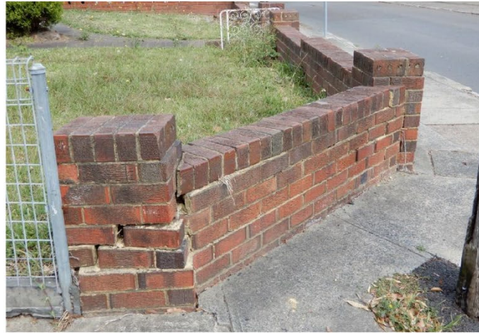
Figure 18: the brick front fence shows uneven settlement and likely impact damage.
