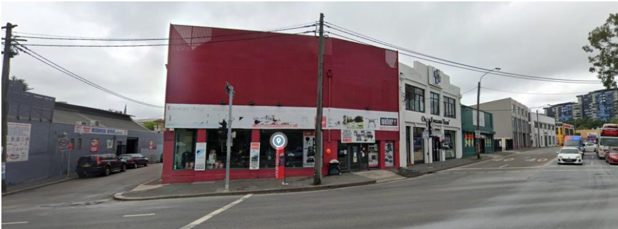
Figure 3 LV overhead asset – Corner Parramatta and Pymont Bridge Roads
