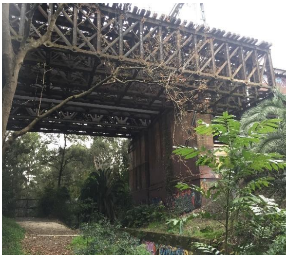
Figure 10: Whipple truss view north from Rail owned land at the southern end of Cadigal Reserve
