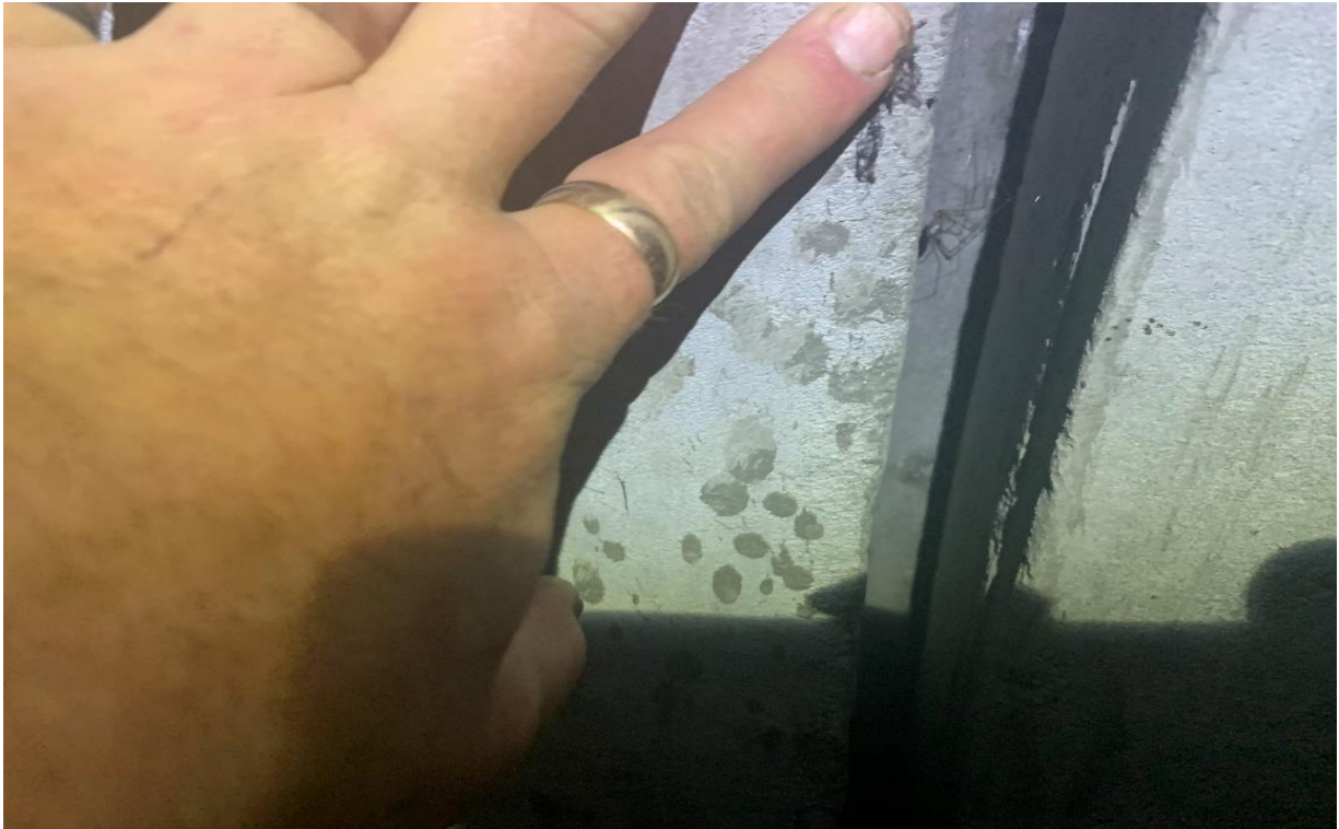
Photo 7: Pipe join between pipe cells in a reinforced concrete pipe culvert that could provide roosting habitat for Large Bent-winged Bats and other subterranean roosting microbat species
