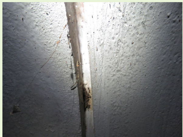
Roof of culvert showing discolouration
