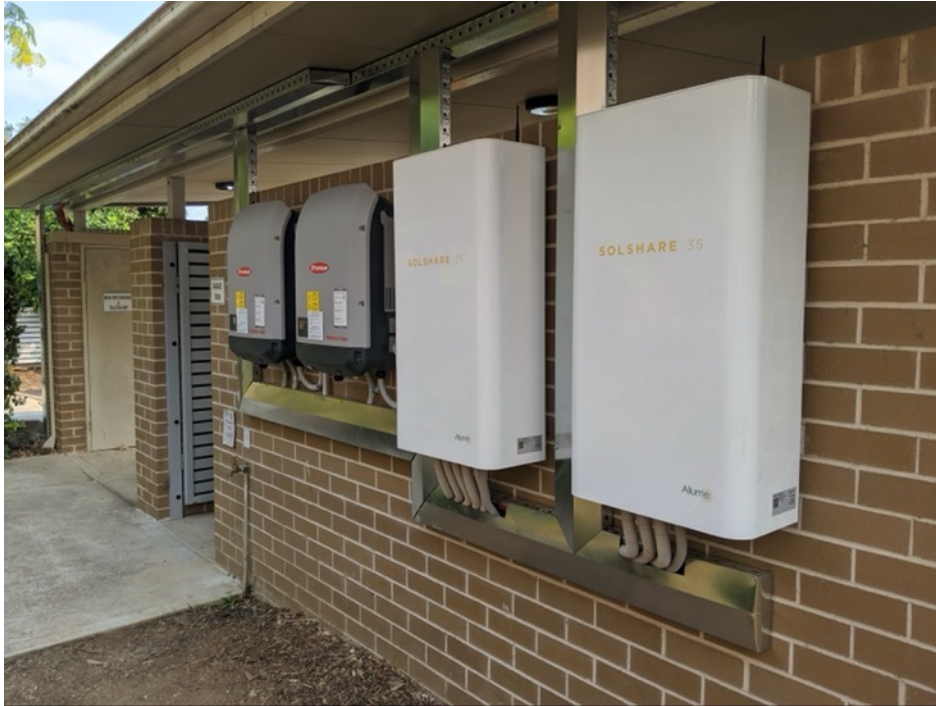
13-19 Warren St Ryde has two inverters and two solar sharing gateways for 17 apartments. Each solar sharing gateway has maximum of 15 apartment connections.
