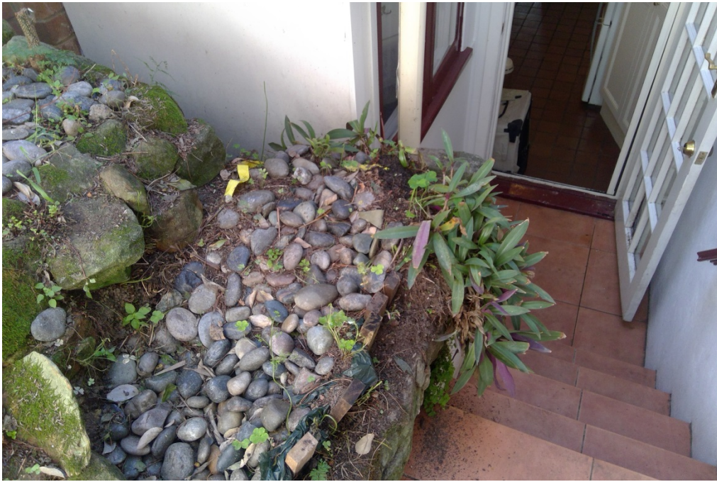
Figure 3: Existing rear ground floor of dwelling with ground floor bathroom and stairs to rear yard.
