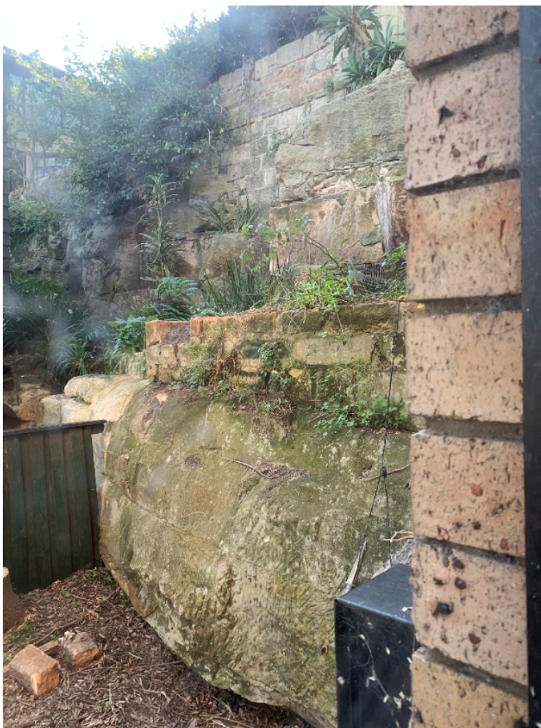
Affected rockface at rear of site.
