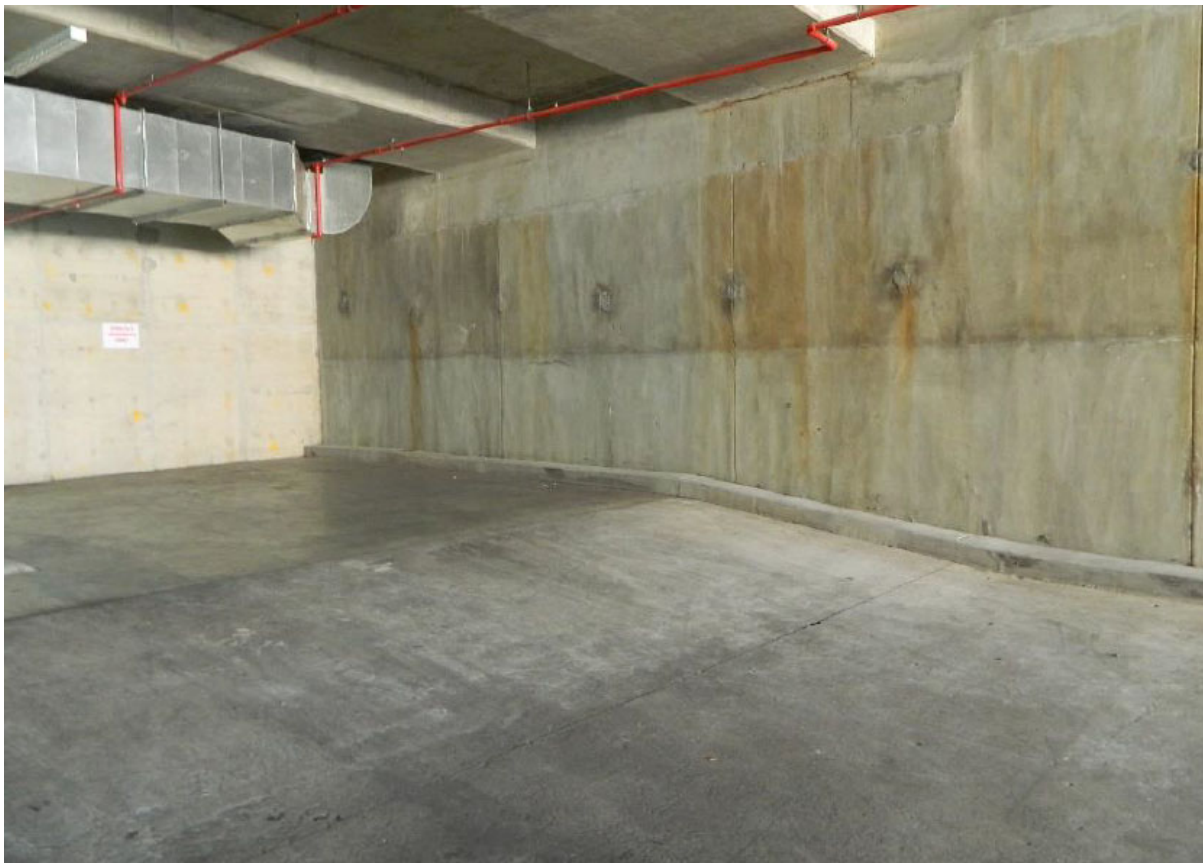
Figure 8: Portion of existing basement wall of No. 1-7 required to be demolished/altered to provide access to subject site.
