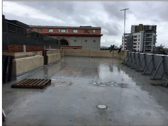
Figure 16: View across roof terrace from west to east. Additional parapet bracing, providing support to the southern parapet, is noted to the right of the image.
