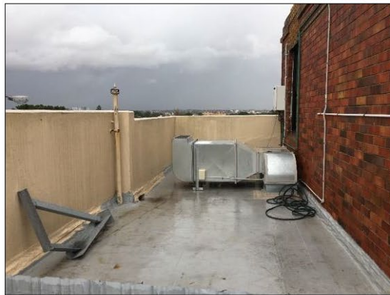
Figure 17: Western most point of the roof terrace currently used to house air conditioning units.
