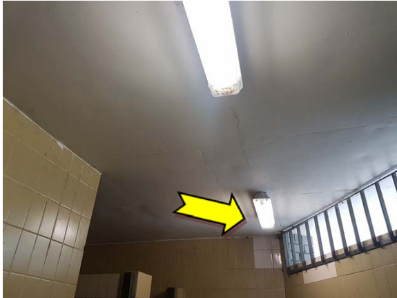
Photo 1. Interior, throughout, single tube fluorescent light fitting – suspected non PCB-containing capacitors.
