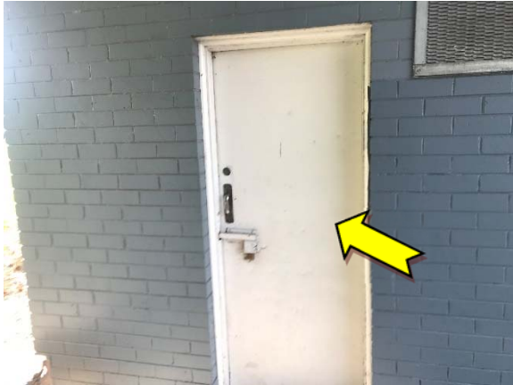
Photo 1. Exterior, throughout, doors and window frames – suspected lead-containing white upper paint system.
