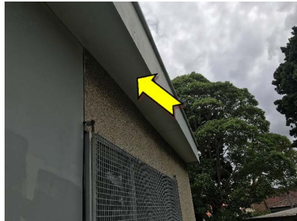
Photo 4. Exterior, throughout, eaves – suspected lead-containing white upper paint system.
