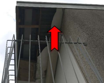
Photo 1. Exterior, throughout, eaves – asbestos-containing fibre cement sheeting.
