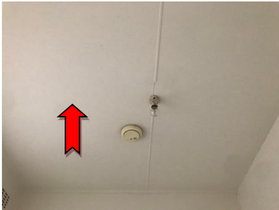
Photo 3. Interior, kitchen, ceiling – asbestos-containing fibre cement sheeting.
