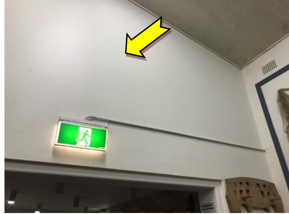
Photo 8. Interior, throughout, walls – suspected lead-containing white upper paint systems.
