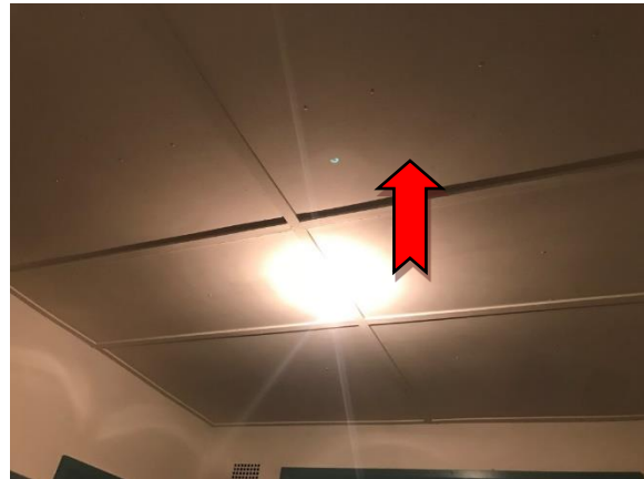
Photo 4. Interior, store, ceiling – assumed asbestos-containing fibre cement sheeting.
