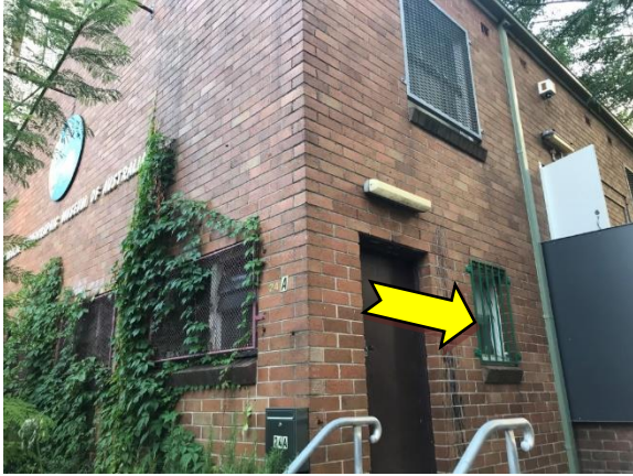
Photo 7. Exterior, throughout, window frames – suspected lead-containing white upper and light yellow lower coloured paint systems.
