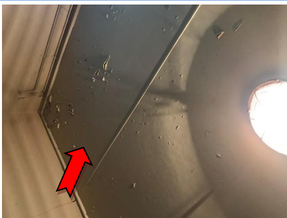
Photo 5. Interior, basement level, store room, ceiling – asbestos-containing fibre cement sheeting and suspected lead-containing cream upper paint system.
