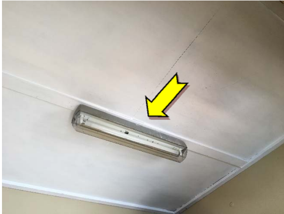
Photo 7. Interior, throughout, single tube fluorescent light fittings – suspected PCB containing capacitors.
