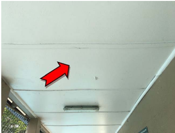
Photo 3. Exterior, ground level, awning – asbestos-containing fibre cement sheeting.
