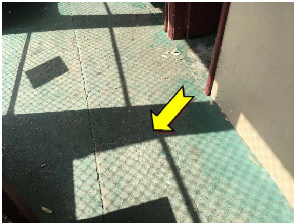
Photo 9. Exterior, throughout, floor – suspected lead-containing green paints system.
