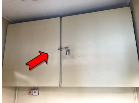
Photo 2. Interior, ground level, electrical backing board – suspected asbestos-containing bituminous backing board.
