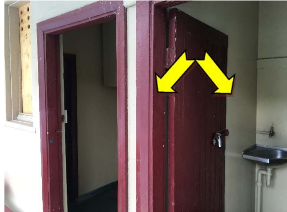
Photo 8. Interior, throughout, walls – suspected lead-containing beige and red paints systems.
