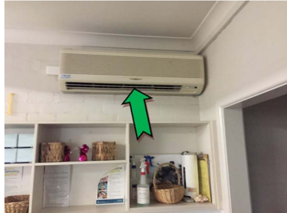
Photo 14. Interior, throughout, Sanyo air conditioning unit – suspected non ODS-containing unknown refrigerant.
