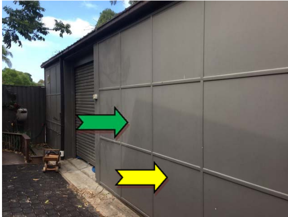
Photo 1. Exterior, east elevation, wall – non asbestos-containing fibre cement sheeting and suspected lead-containing grey upper paint systems.
