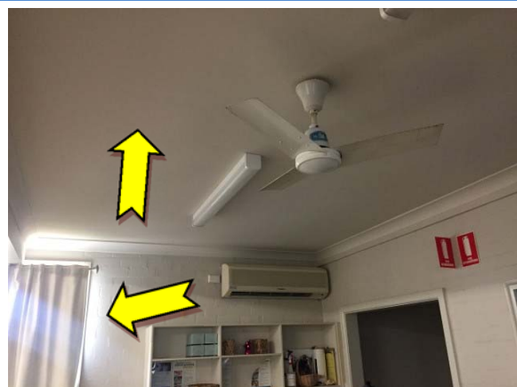
Photo 12. Interior, throughout, walls and ceiling – suspected lead-containing beige and white upper coloured paint systems.
