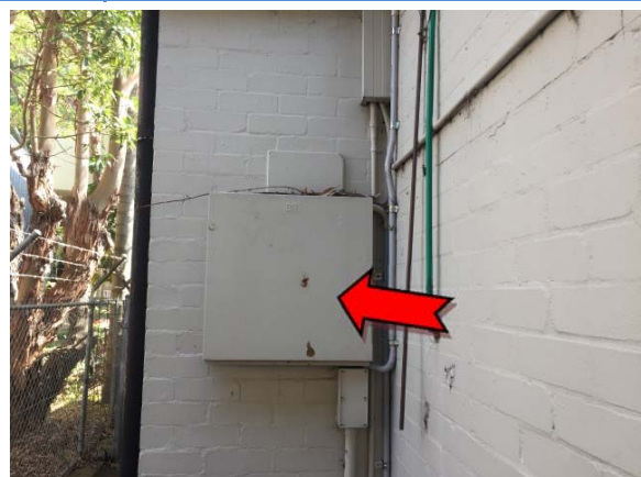
Photo 6. Exterior, south-west corner, electrical backing board – suspected asbestos-containing bituminous backing board.
