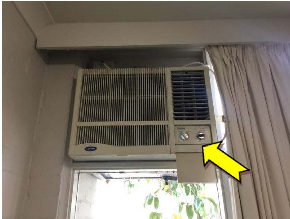
Photo 13. Interior, office, air conditioning unit – suspected ODS-containing unknown refrigerant.
