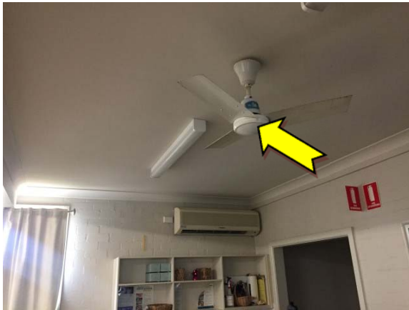
Photo 15. Interior, family room, ceiling fan – suspected PCB-containing capacitor.
