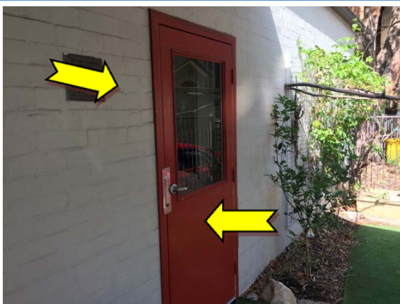
Photo 11. Exterior, throughout, walls and door – suspected lead-containing cream and red upper coloured paint systems.
