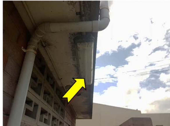
Photo 2. Exterior, throughout, double tube fluorescent light fitting – suspected PCB-containing capacitor.
