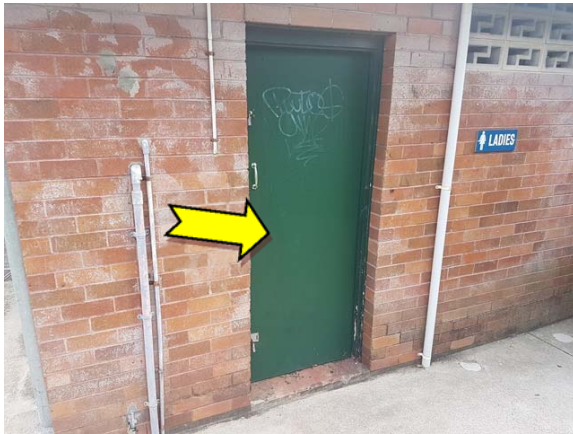
Photo 3. Exterior, throughout, doors and door frames – suspected lead-containing upper green paint system.
