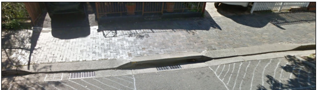
Image 4: Similar crossing nearby with re-laid bricks at Victoria Road (which also forms part of I98)
