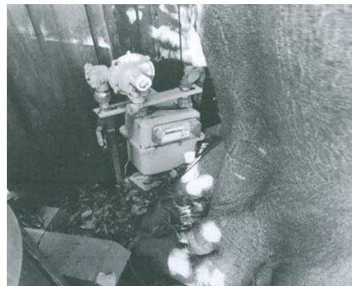
Figure 6: Trunk of the subject tree pressed against gas meter and main
