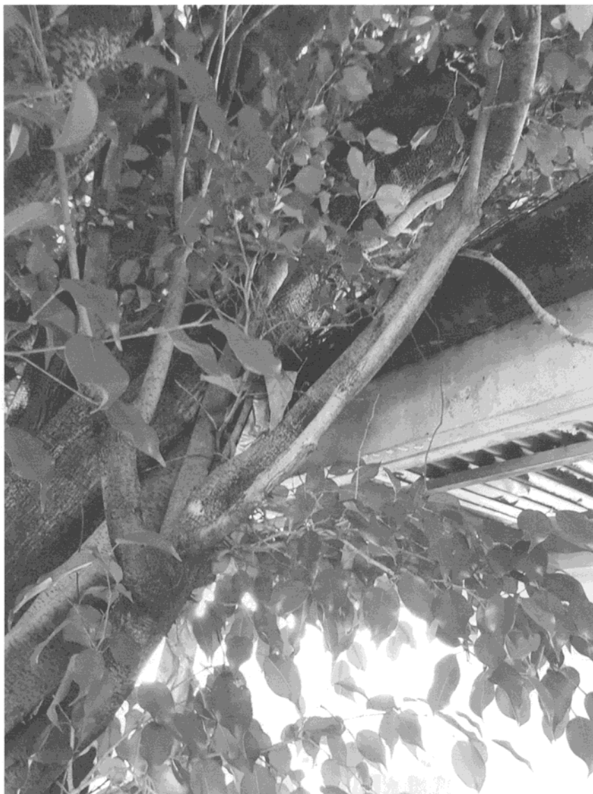
Figure 2: Damage to guttering that cannot be corrected through pruning.
