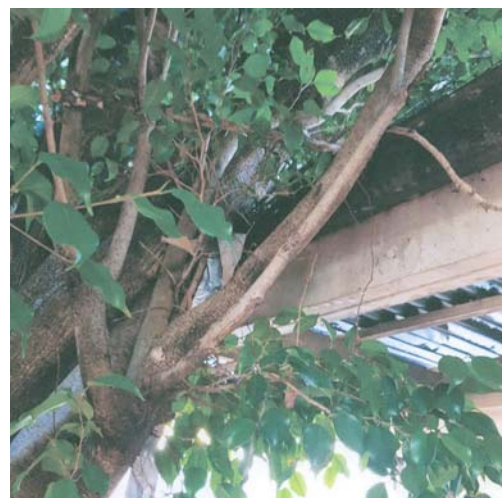
Figure 8: Branches pressed against the gutters of the building
