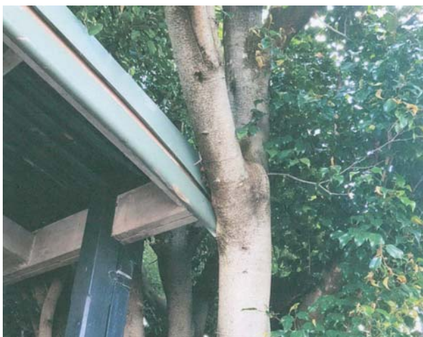
Figure 7: Branches pressed against the gutters of the building
