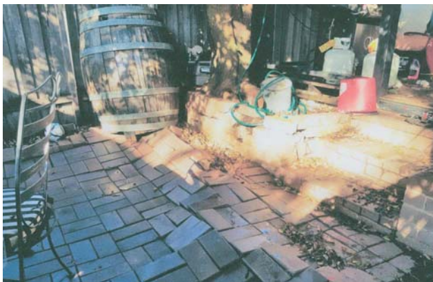
Figure 5: Raised paved areas caused by large extending roots
