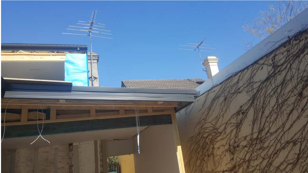
View of the subject rear roof plane from the backyard of the adjoining property at No. 11 Reserve Street.
