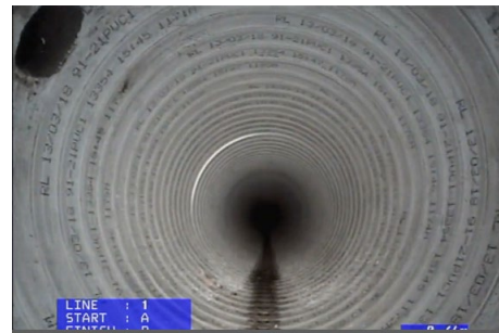
Example of “after”
