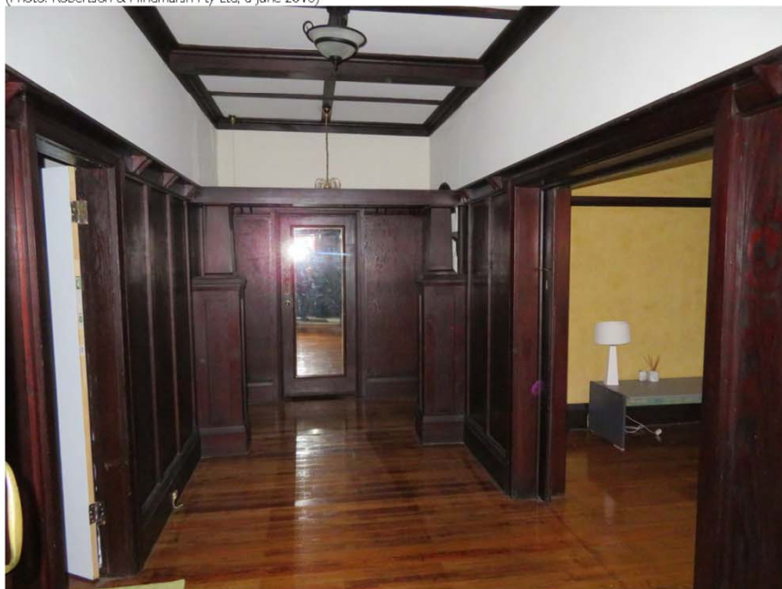
Figure 3.6 No. 73 The Boulevard, Dulwich Hill: Main (cross) hall looking north past Living Room doors on right to Bedroom at end of hall (Photo: Robertson & Hindmarsh Pty Ltd, 6 June 2018)
