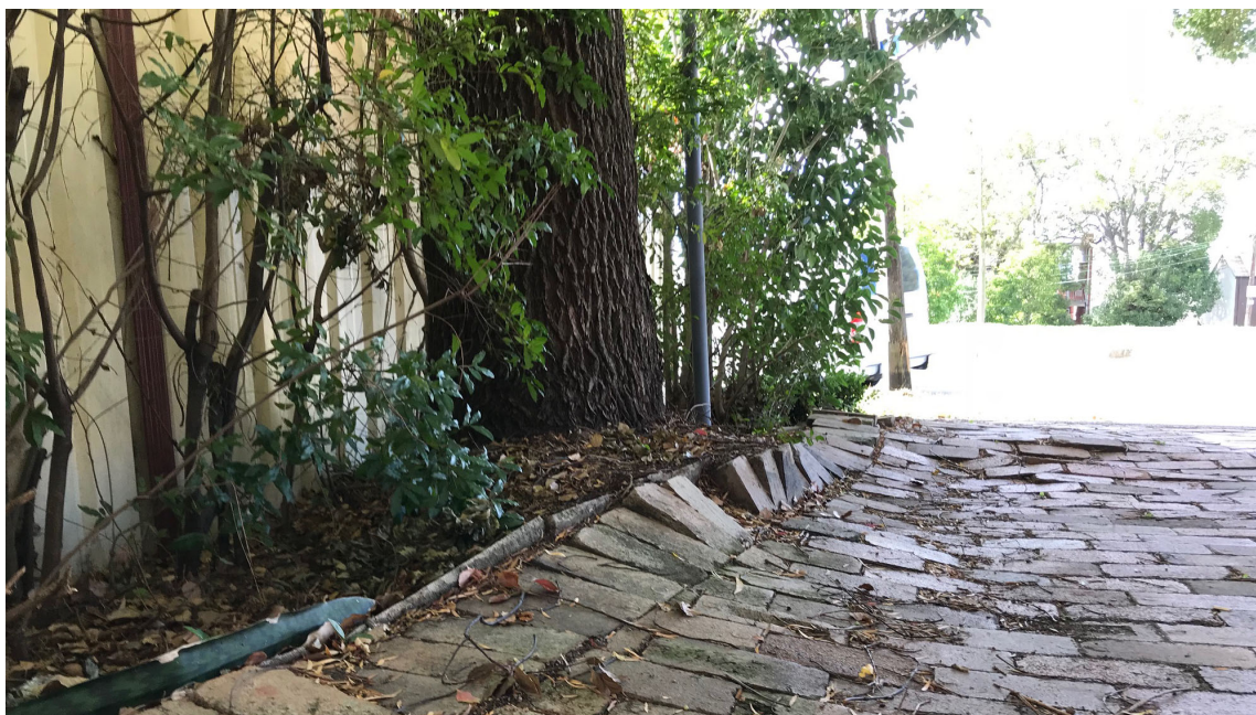
Photograph of the Camphor Laurel tree at the front of the property showing damage to paving.
