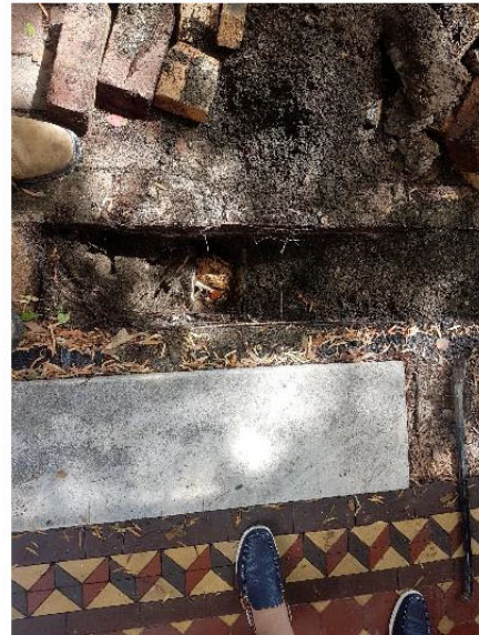
Fig 6. Excavation and tree root beside Mr. Zhang's verandah.
