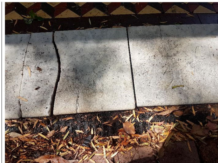
Fig 7. Cracking and uplift to tiles on Mr. Zhang's verandah
