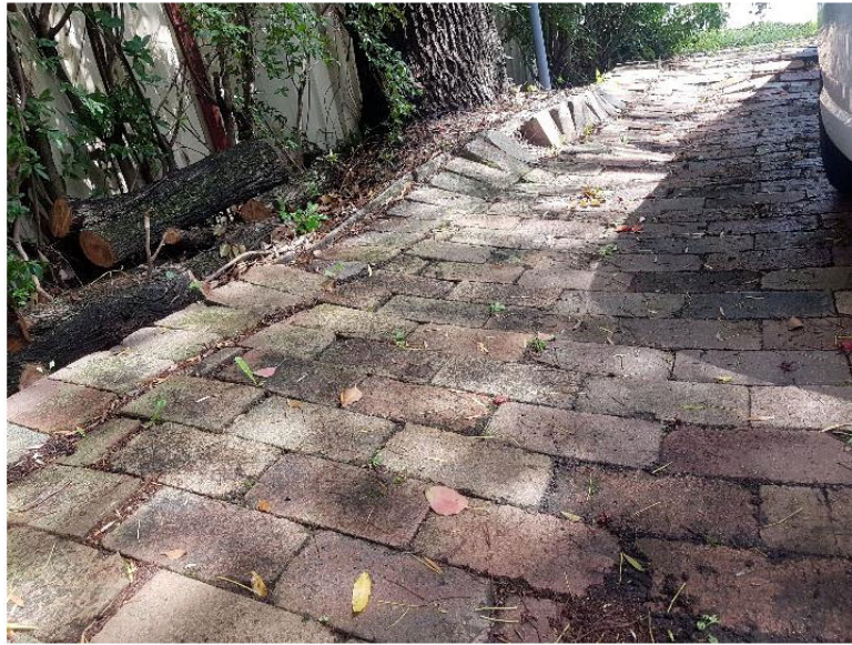
Fig 8. Up lift and displacement of Mr. Zhang's driveway pavement.
