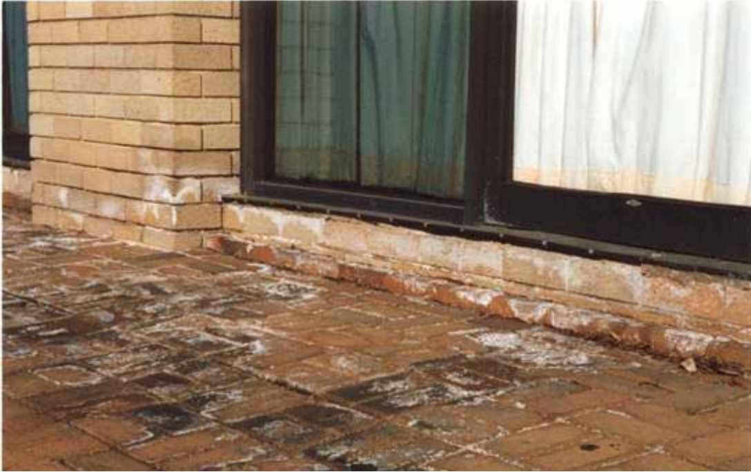
A salt-damaged public building in Western Sydney
