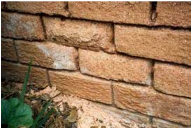
Fig 2: Salt-affected buildings in Western Sydney
