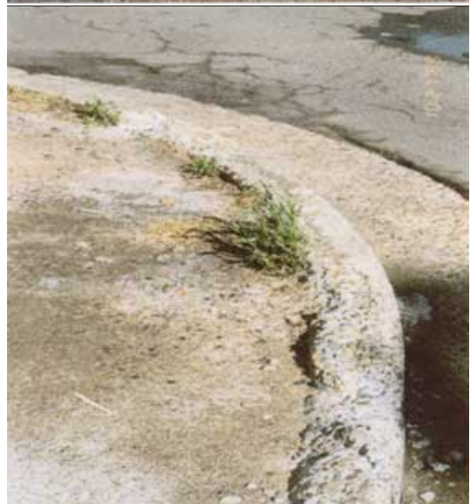
Fig 3: Salt-affected roads in Western Sydney
