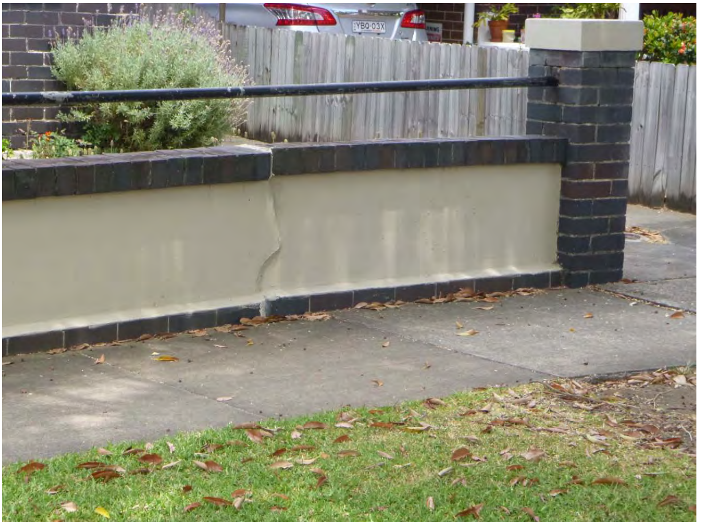
Figure 2.26 - Trees can cause issues, but in many instances these are relatively minor and can be managed without tree removal. When damage is to minor or ancillary structures such as landscape walls, the retention of the tree should be given priority using some of the strategies listed in Table 5. (Photo-Artterra)
