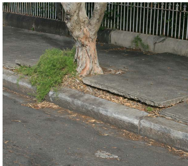
Figure 1.14 -Infrastructure damage is one of the most common impacts of street tree planting (Photo Arterra)
