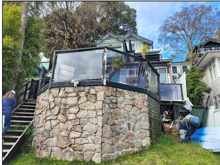
Figure -1: view from rear garden looking onto the existing dilapidated pool deck (Source: Sky Planning)
