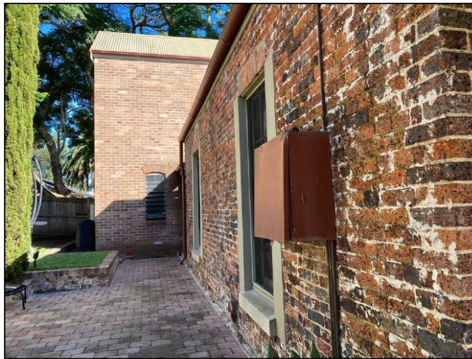
Figure 13: Southern elevation to the principal building, also showing part of the rear addition.
