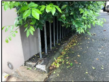
Figure 26. Iron palisade fence and sandstone base to Wharf Road boundary of subject site.
